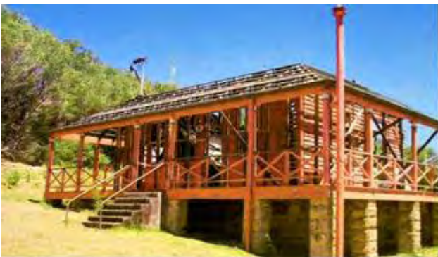
BUILDING P22 FOLLOWING FIRE (OCT 2001)
