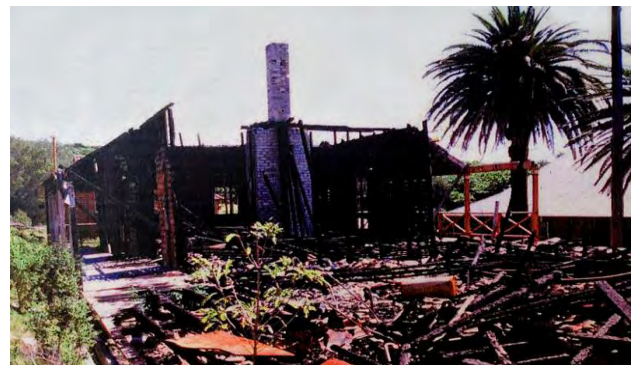
BUILDING P22 FOLLOWING FIRE (OCT 2001)
